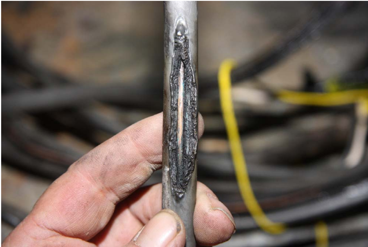
F08-049: Localized Melting at the Grounding Conductor
