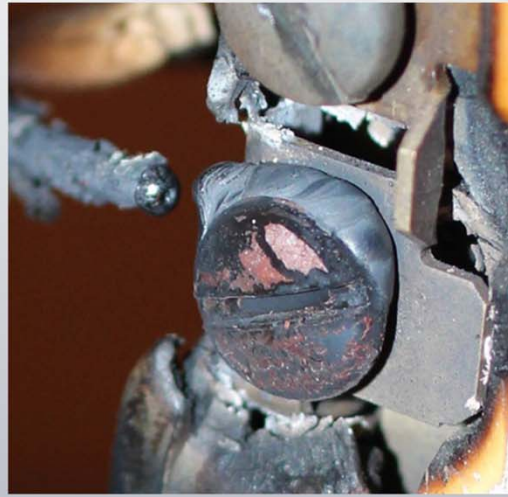
Severed Conductor (Welded w/Curved Striations)
