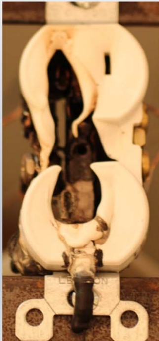
Melting, running and dripping
